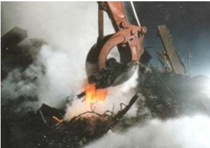
Figure 2: An excavating machine at Ground Zero lifts debris dripping with molten metal.
